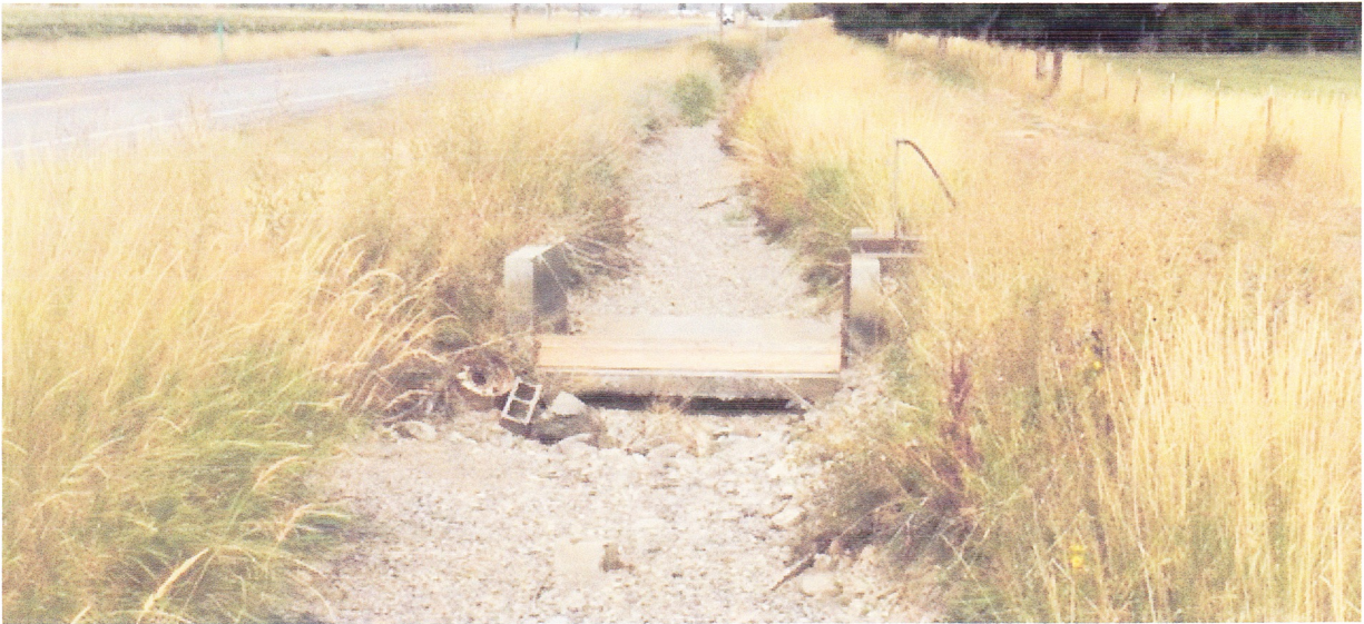
This photo stirs up the debate: where does the District's responsibility stop and the user's responsibility start? Just to clarify: the cement structure is owned and maintained by the user. But who is responsible for the dirt underneath and the banks immediately surrounding the structure, which are being effected by a combination of the structure and the water? It seems trivial....until it isn't...
