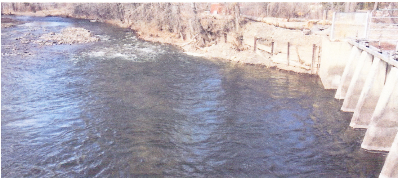
Keith removed the remainder of the dam this afternoon. Now there is 24" of water awaiting against the Main Gates. This is our first chance to see if our new floors, put in last Fall, gave us a little more positive control on shutting down the gates.
